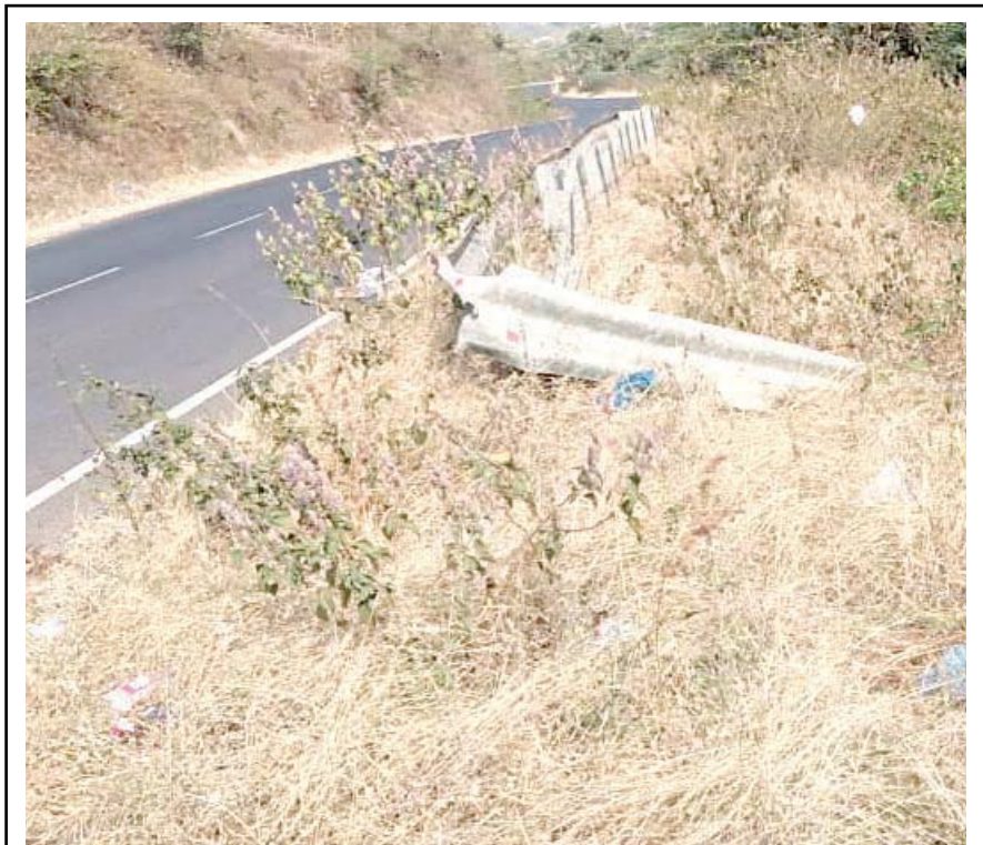
Barricades and direction boards on the Nashik-Surat-Saputara-Wani national highway are in poor condition, especially at Saputara, Thanapada, Hatgaon, and Borgaon. With heavy traffic due to major vegetable markets in Nashik, Surat, Ahmedabad, and Ankaleshwar, the deteriorated signage and barricades increase the risk of accidents. Concerned drivers have demanded that the Public Works Construction Department should take immediate action to repair them.
