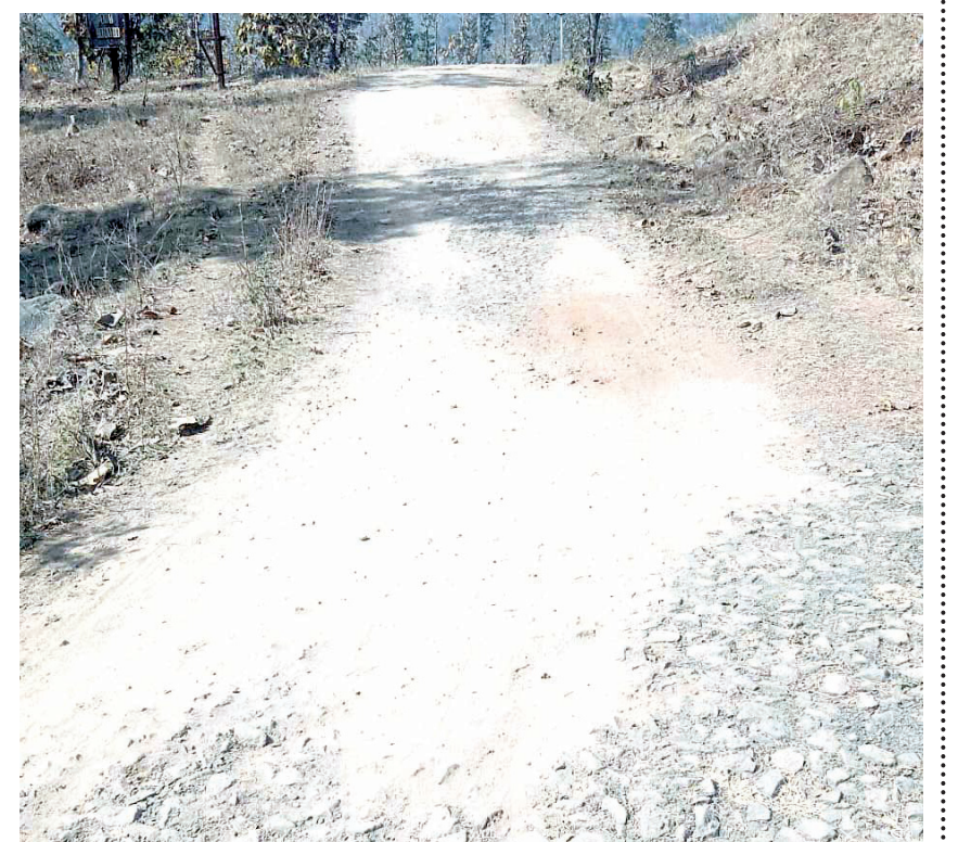
The Dabadi-Kopurli route in Peth Tehsil of Nashik district is in a severely deteriorated state, making travel extremely difficult for drivers and commuters. This has led to significant inconvenience for daily travellers, including students, workers, and residents of nearby villages who rely on this route for transportation. The demand for road repairs has been growing, as the current state of the route is causing unnecessary delays and hardship for people who use it regularly.
